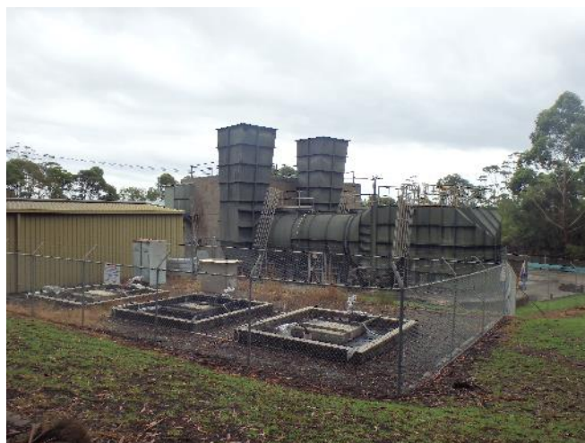
Example of a site where redundant transformers were removed following incidents at other sites
