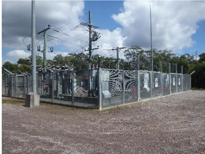
Example of a transformer yard associated with a large vent shaft site in the Special Area
