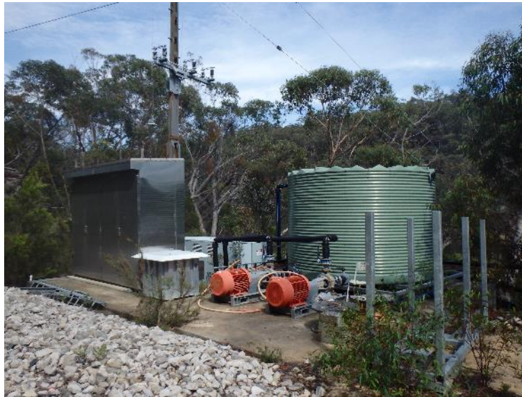
Example of a pump station site adjacent to Cataract Dam
