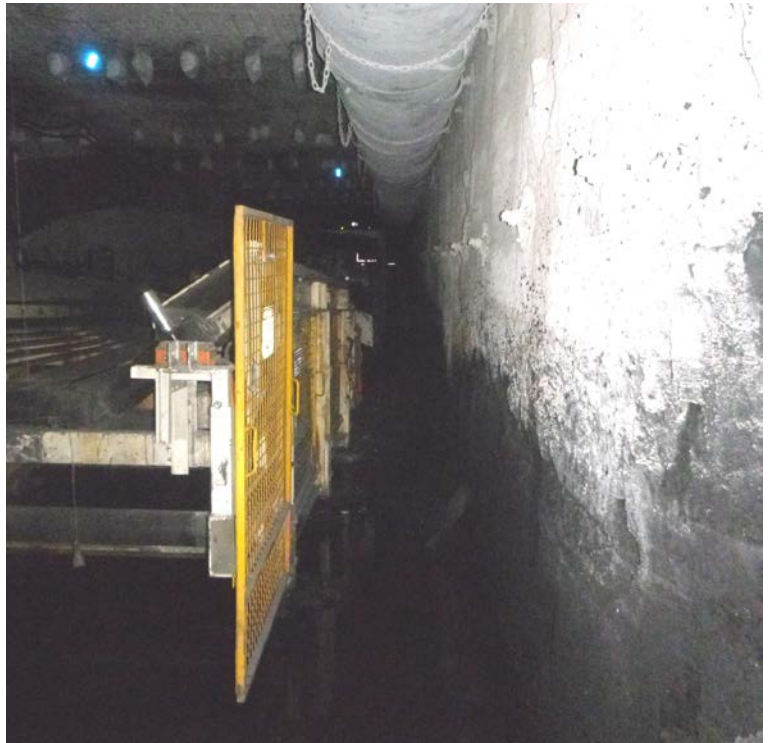
Figure 1 The boot end where the worker was injured
