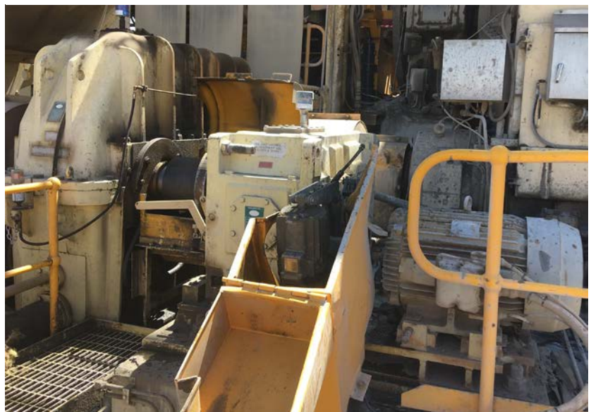
Figure 1 The drive assembly showing two gearboxes (left and right), motor and failed brake assembly
