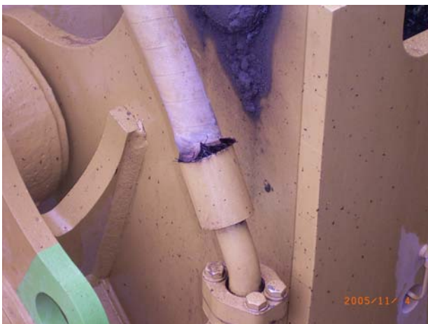
Corroded hose end
