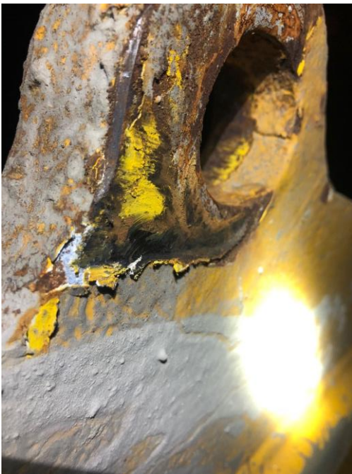
Figure 4. Gouge marks on face of workbox locking pin receptacle
