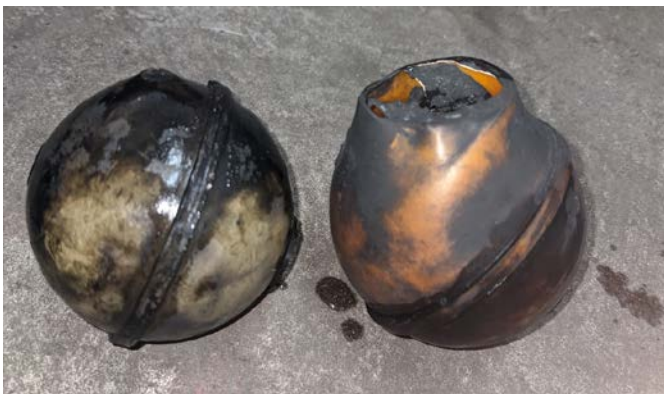
Figure 1 Heat-affected scrubber floats
