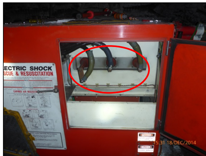
Figure 2: Opened test compartment on IS43. Test points circled
