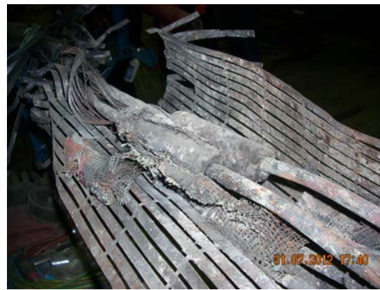
Figure 2: What remained inside the cable splice cage.
