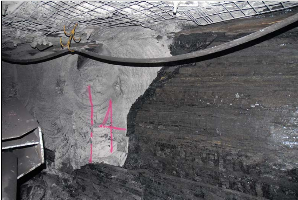
Photograph 9 View rib showing the two bolt and plates in the white stone dusted area prior to the fallen area.
