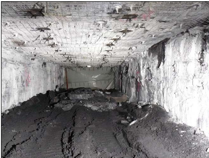
Photograph 22 Looking inbye in D Heading showing a large rib slab on the floor in the centre of the photo, which appears to have come from the removal of a rib slab on the night shift before the incident.
