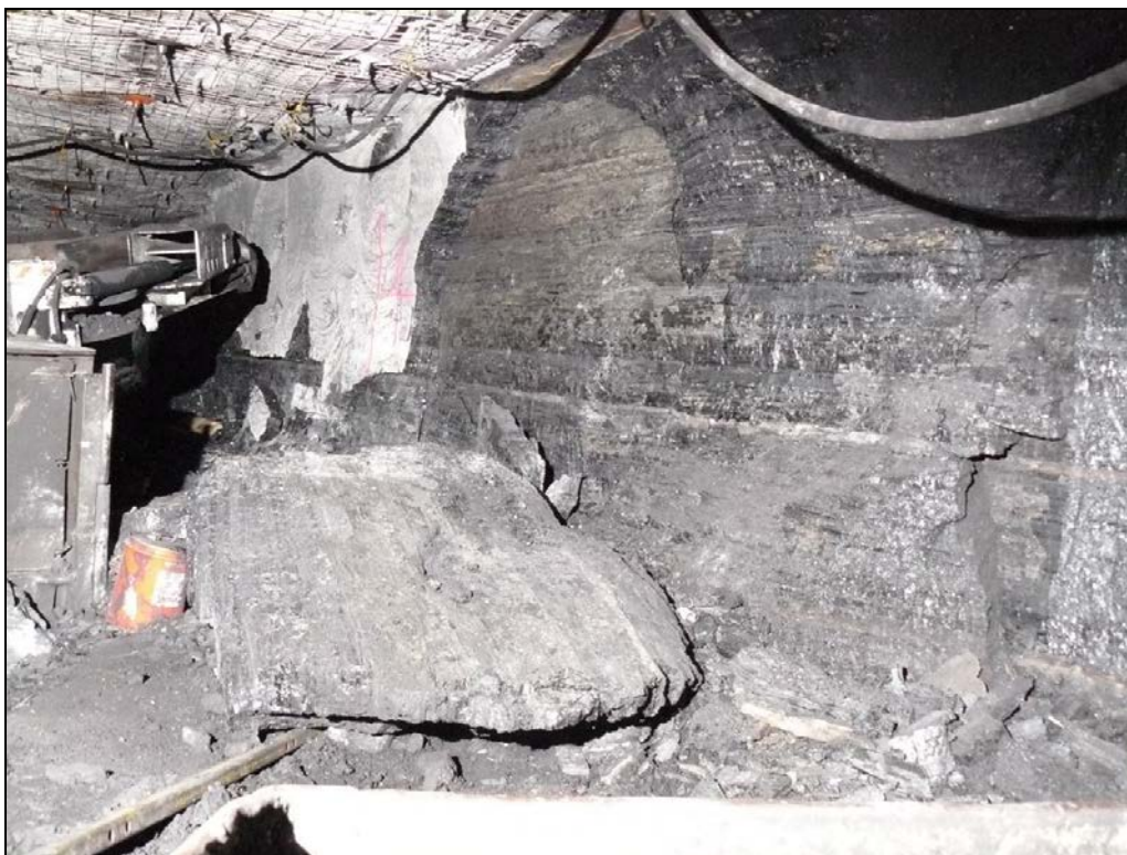
Photograph 8 View of the incident scene on Saturday 4 June 2011 looking towards the area of rib slabbing and rib slab on ground. Photograph taken inbye of the continuous miner. Note the red oil drum and steel belt clamp used in the rescue of Mr Jones.
