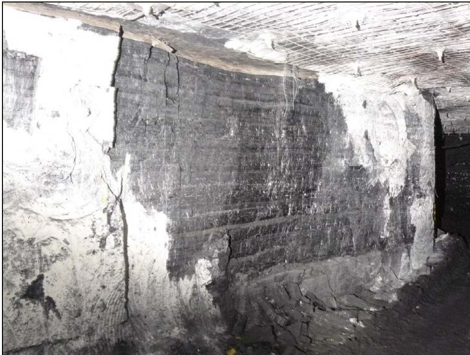
Photograph 23 Looking inbye in D Heading showing a large unsupported area of rib side in a shuttle car wheeling road.
