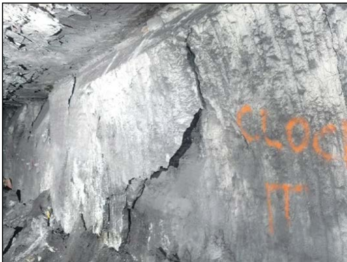
Photograph 1 Looking at 5 cut-through of the left hand rib noting that significant deformation and failure in the rib side and that the rib does not contain any rib bolts. Also note that a person has painted the words "CLOCK IT" on the rib to identify the placement of a roof monitoring device.
