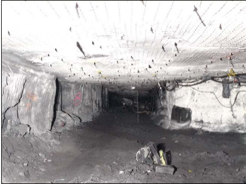
Photograph 21 Looking inbye at 5 cut-through of the left hand rib noting that a significant distance of rib does not contain any rib bolts.
