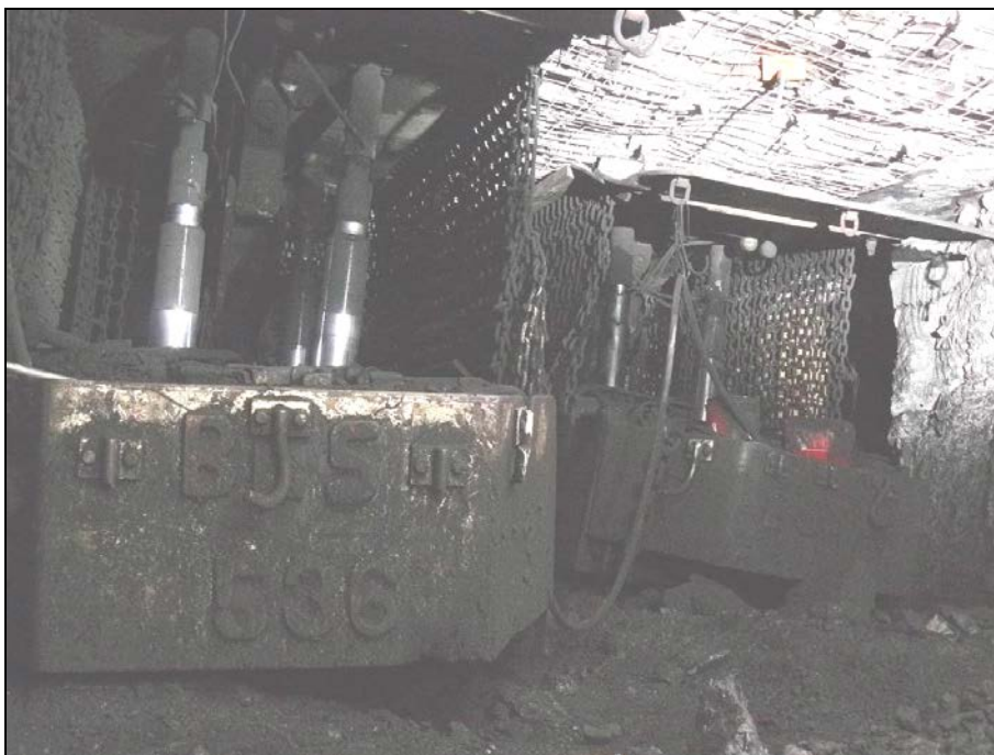
Photograph 14 Looking inbye showing the position of the 2 breaker line supports in B Heading.
