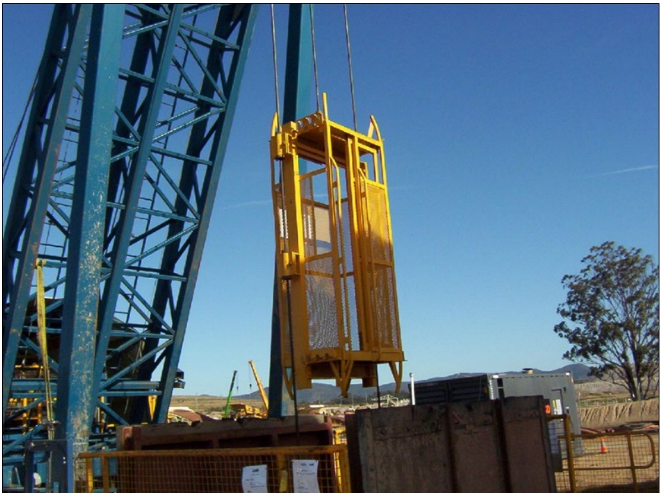
Figure 10 Shaft sinking winder cage
