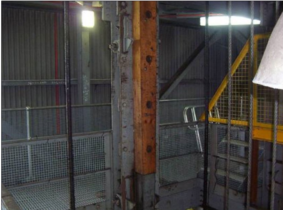
Figure 23 Wooden arresting device and safety catches
