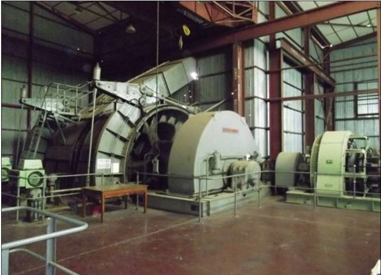
Figure 2 Ground mounted, vertical shaft double drum winder
