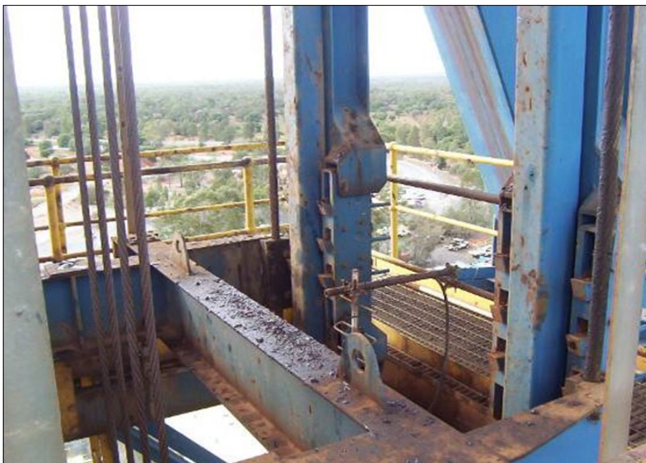
Figure 22 Headframe safety catches
