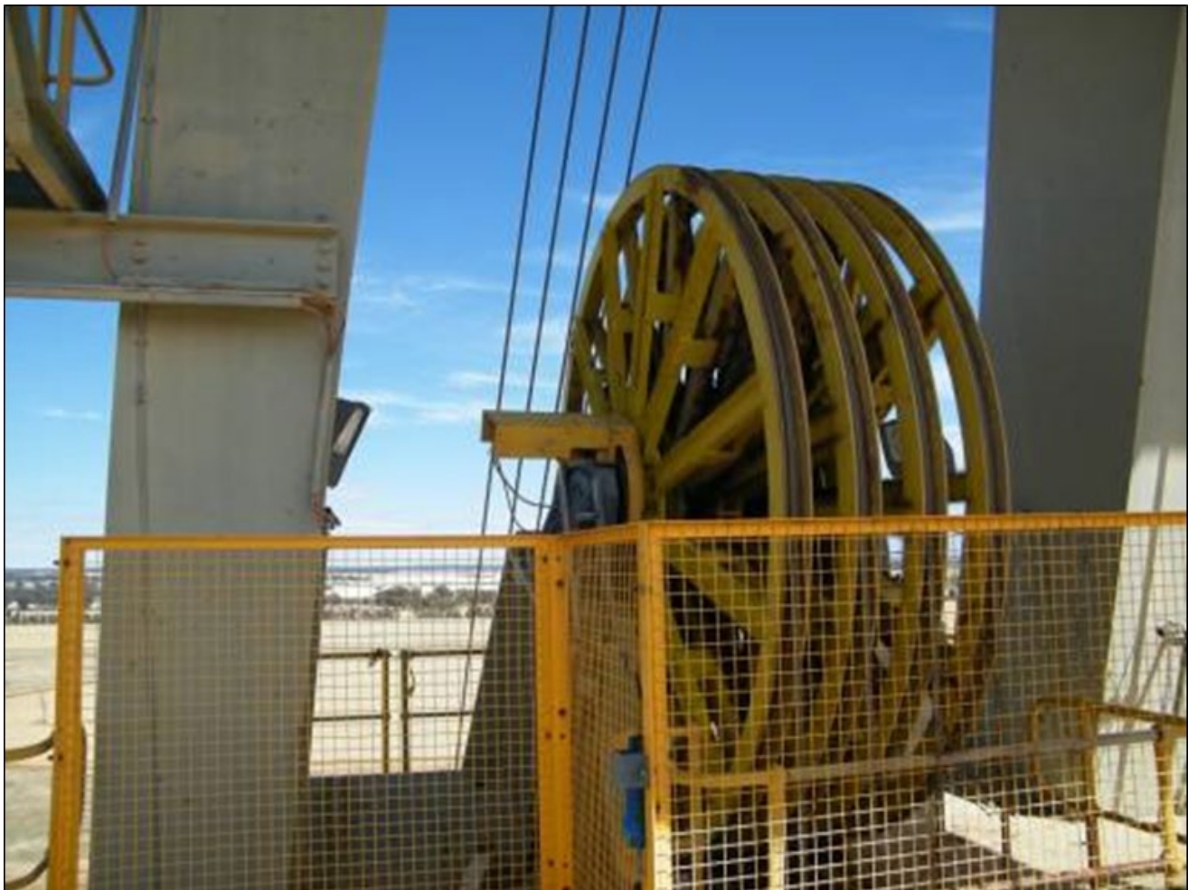
Figure 27 Headframe mounted friction winder headsheaves
