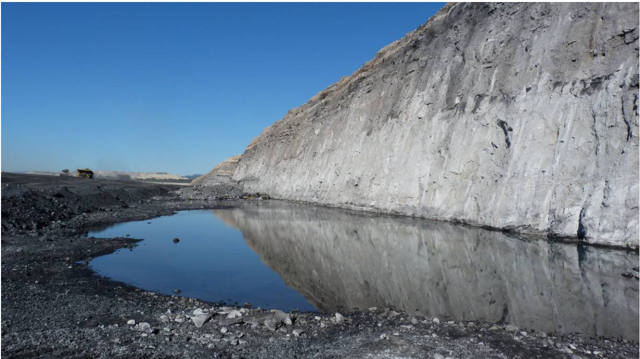
Photograph 5: Water spread across the coal bench at Moorlands Pit (view looking south).
