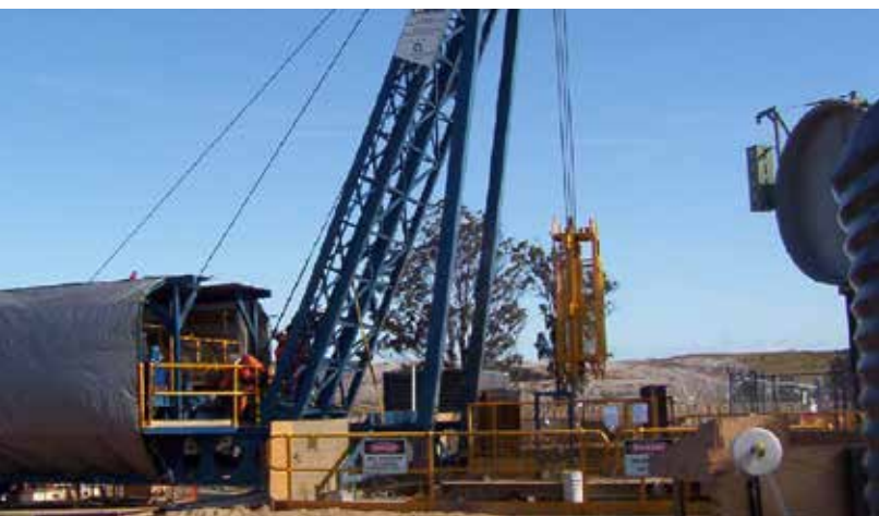
A shaft sinking winder on a NSW mine site.
