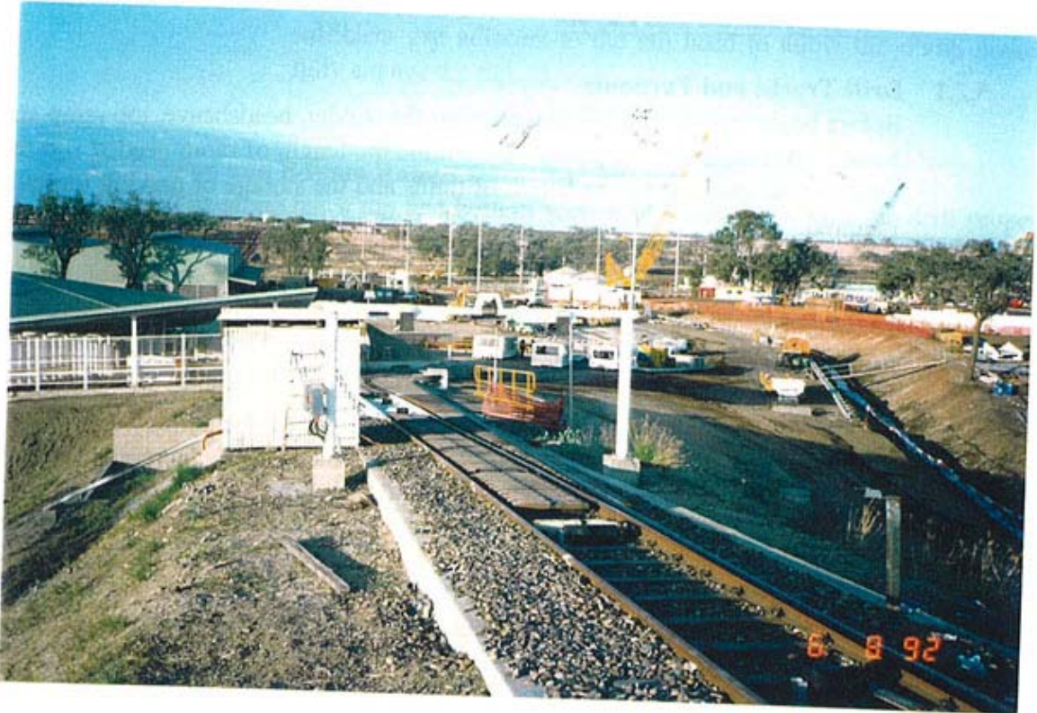
Top Ramp Track - 1 in 10 Gradient
