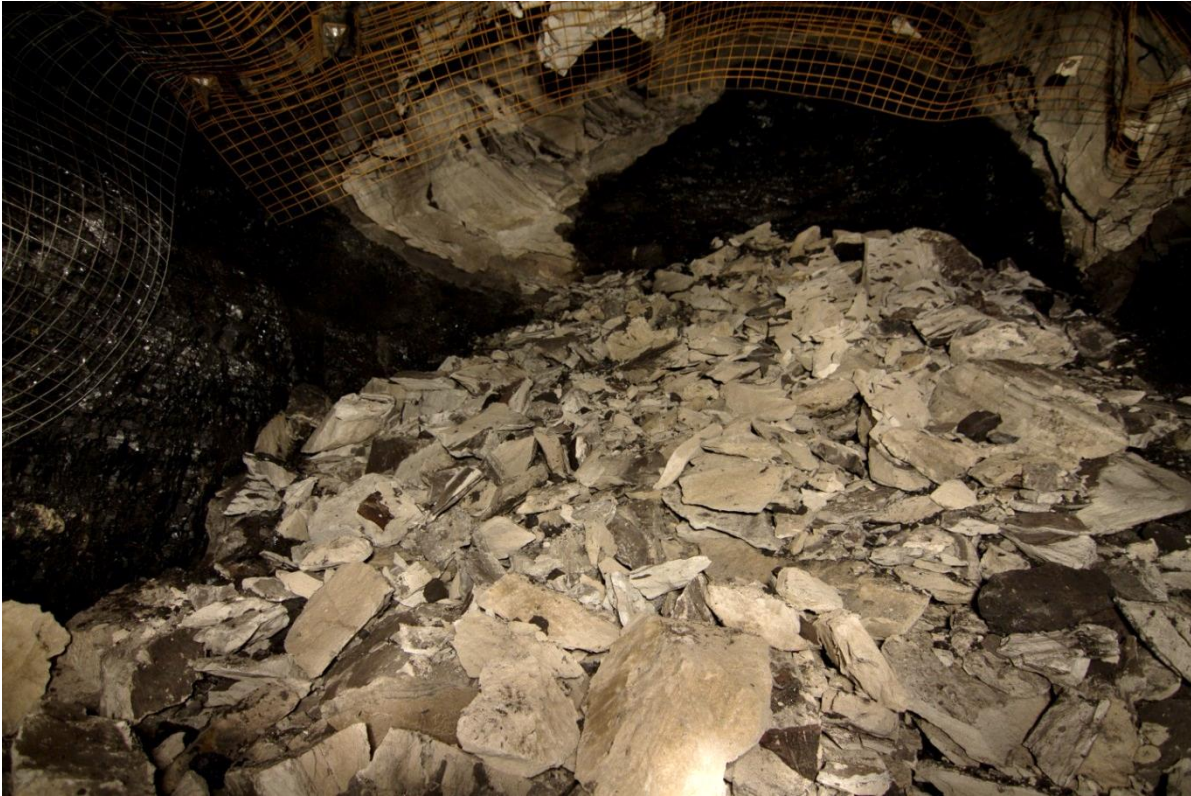
Figure 6 Heading A face, intersection with the unanticipated fault.
