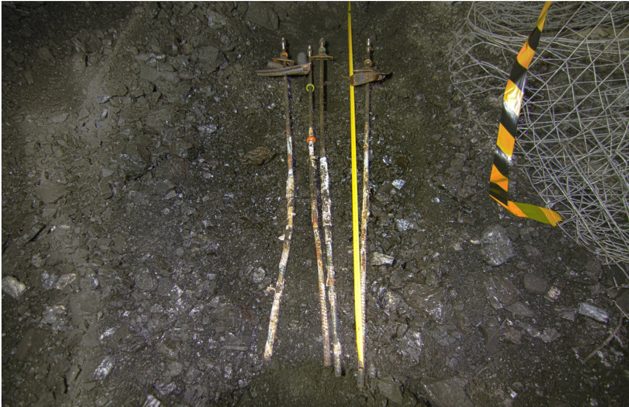
Figure 23 The chemical anchor bolts removed from the incident scene. Note each bolt appears to have full encapsulation of chemical resin.
