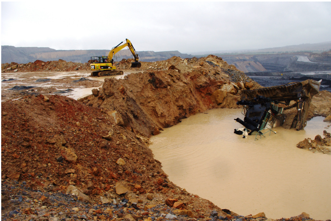
Dozer submerged in the test hole.
