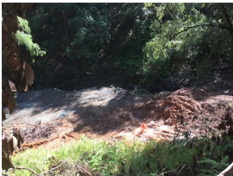
Figure 2 Poor drill cutting management and substandard erosion and sediment controls near a watercourse
