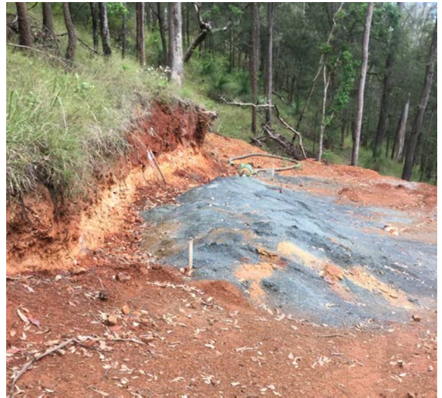
Figure 4 Poor drill cutting management
