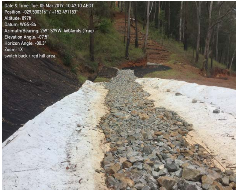
Figure 5 Effective use of sediment and erosion controls, application of vegetation (branches) across slopes
