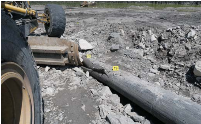
Photograph 2: The grader and the punctured pipeline.
