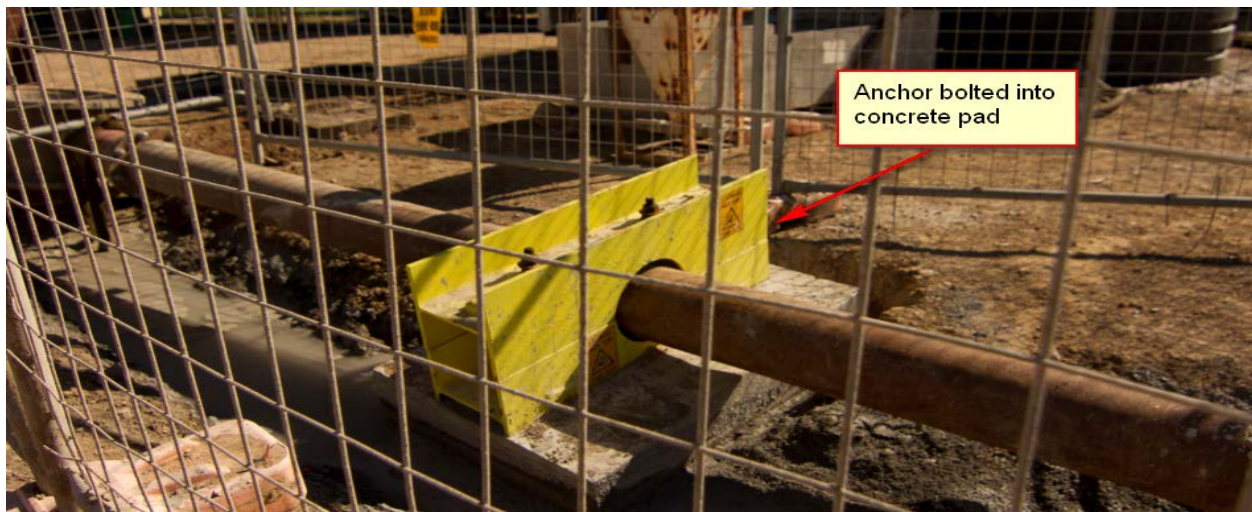
A blooie line anchoring method used at Ashton Coal following the incident
