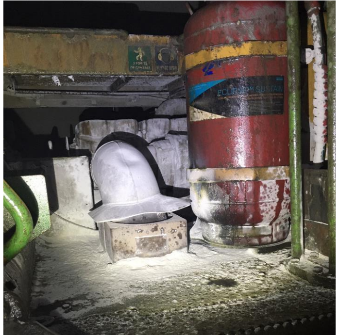
Figure 19. Damaged DPF box and exhaust pipe
