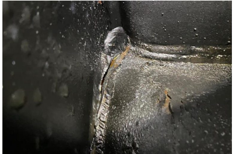
Figure 17. Location of cracked weld
