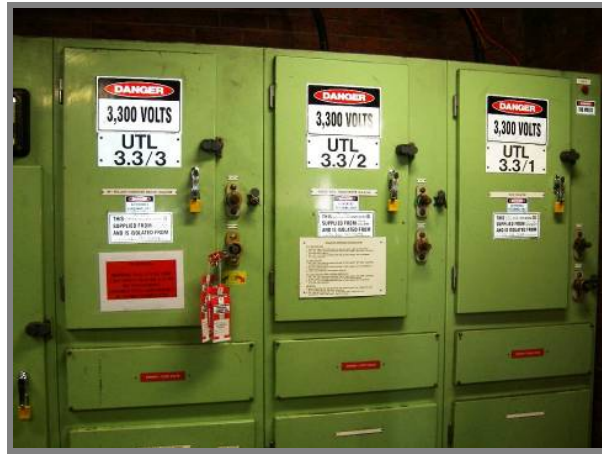
Photo showing 3.3kV switchboard located in UTL building
