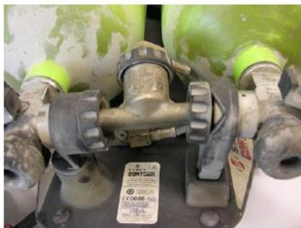
CABA unit showing curved connection - should be straight
