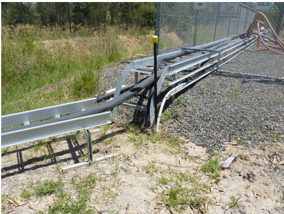
Figure 27: Break in cable tray showing lack of earth bonding
