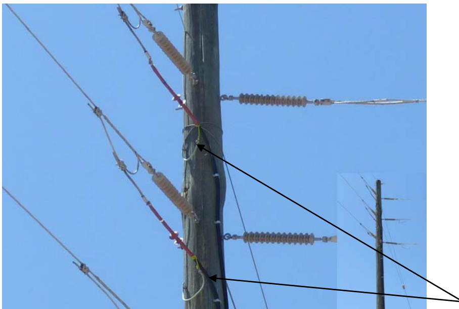
Figure 25 – Photograph showing UGOH pole and earthing wires. Note that the overhead high tension earth is connected to the 11 kV earth.
