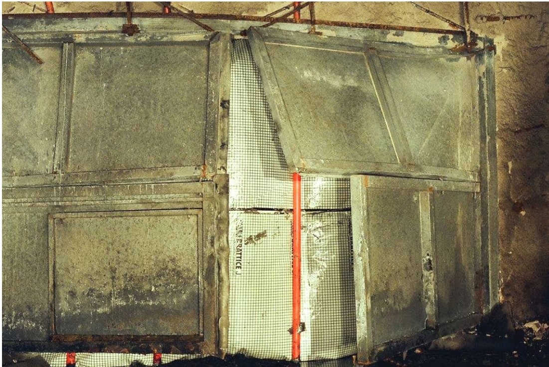
Figure 11 – Double doors at 38 cut-through looking from heading ‘A’ to heading ‘B’ Photograph by Tim Flowers 14 December 2011
