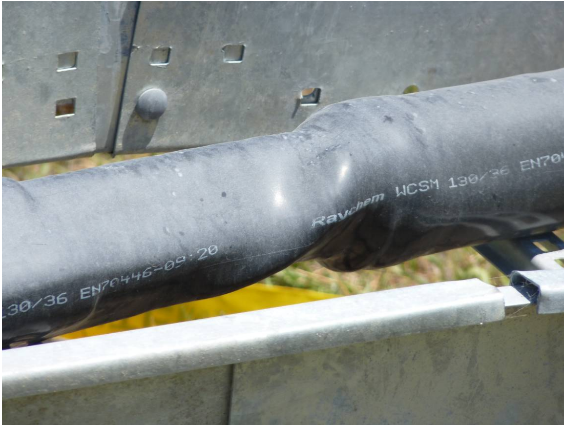
Figure 28 – High tension cable join showing poor quality join
