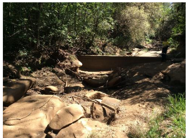
Figure 11 Loss of water in Redbank Creek weir pool
