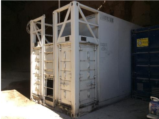
Figure 1 Self-bunded diesel fuel storage tank
