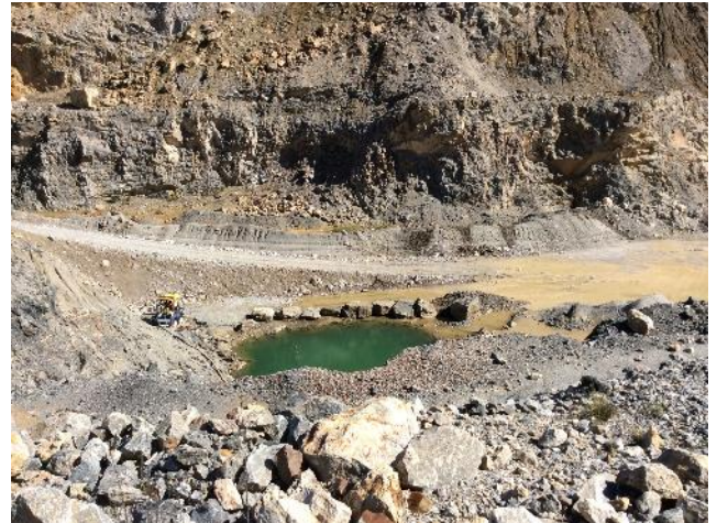
Figure 3 Pump operating to pump water from open cut pit 1 to the wet quarry
