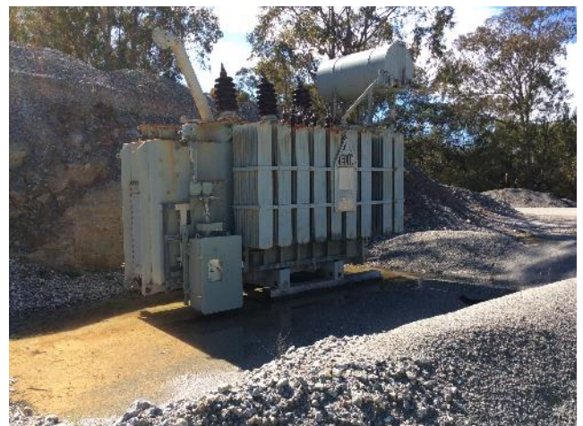
Figure 6 Decommissioned transformer in the product storage area
