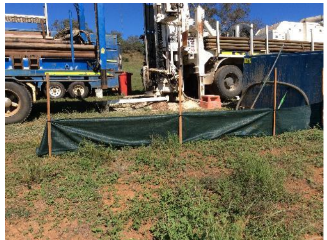
Figure 4 Sediment fencing erected downslope of drill rig and adjacent to aboveground sump at BH22
