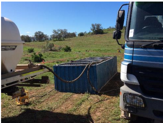
Figure 3 Aboveground metal sump for drilling muds/returned water at BH22
