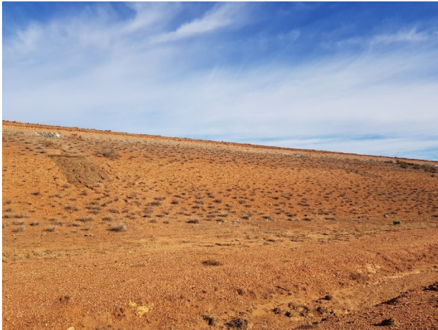
Figure 3 Erosion on the western embankment of the TSF
