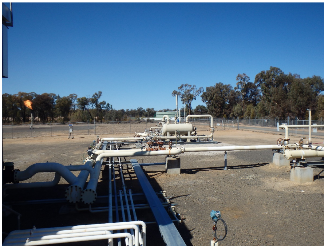
Photo 3: Gas metering and flare at Bibblewindi compressor station.
