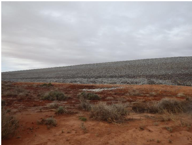
Figure 12 Seepage from possible TSF leak
