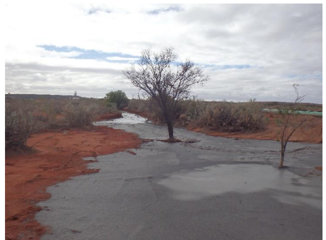
Figure 15 Tailings spillage at Site D TSF
