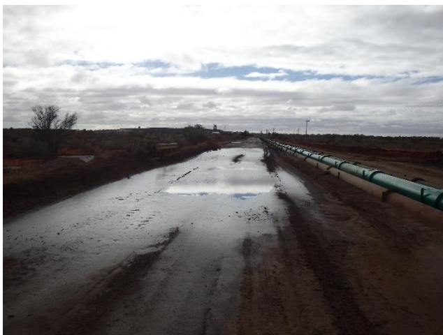
Figure 14 Site of tailings line leak at Site D TSF
