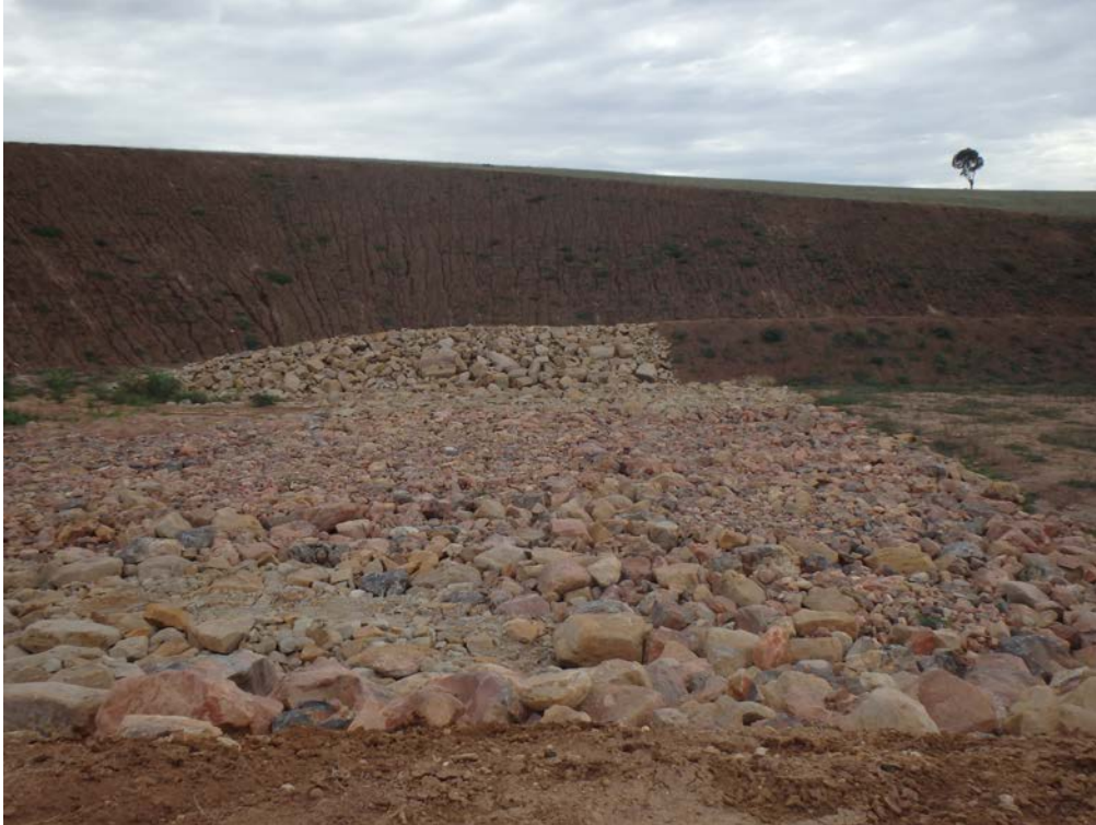
Figure 4 Revegetation failure and erosion on construction batters at the tailings dam
