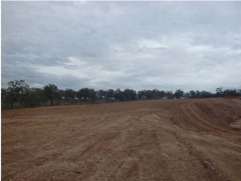
Figure 1 Pit D topsoil stockpile showing no erosion controls on the slope
