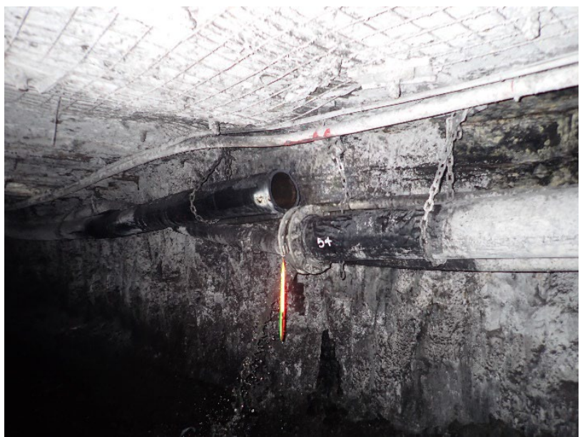
Figure 3: The 250 mm pipe hit by the monorail sled has impacted HV cable
