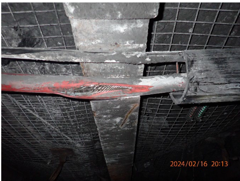
Figure 1: High voltage cable struck by shield carrier
