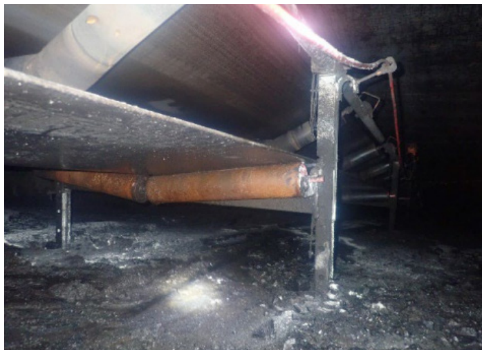
Picture 20. Smoke damage on conveyor structure
