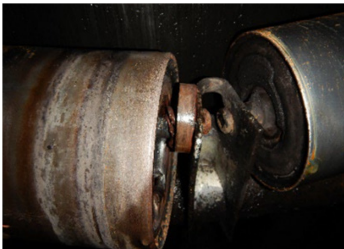
Picture 21. Defective roller involved in fire incident
