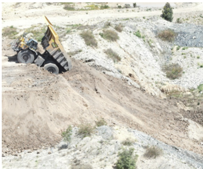
Picture 13. Slumped material and truck
