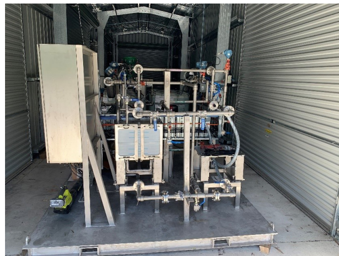
Experimental Forward Osmosis facility ready for acceptance testing at CSIRO in Pullenvale. Two Forward Osmosis modules shown on left hand side of skid. Photo courtesy of CSIRO.
