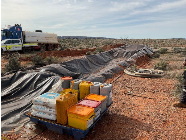
Figure 6: Inground sump at EL6400 hole GR24RC015
