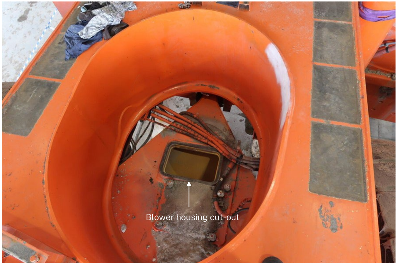
Figure 1: The work area and blower housing cut-out that the worker was attempting to manually manoeuvre the lifting plate through
