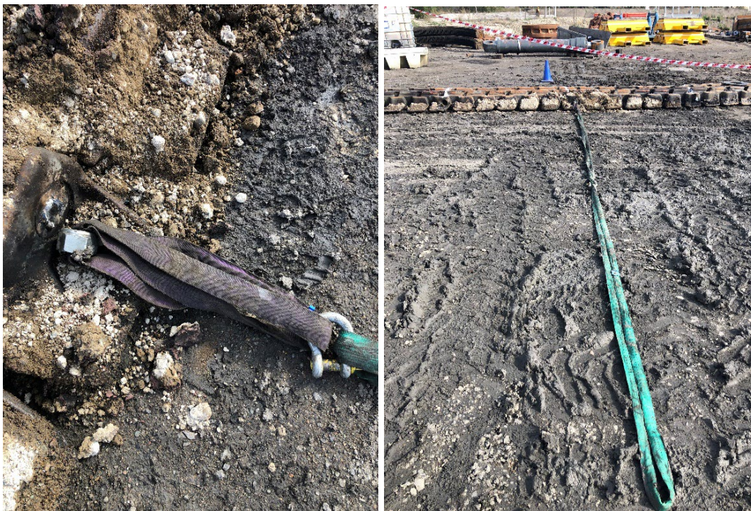
Figure 2 – Sling connection to forklift was re-enacted after the incident
