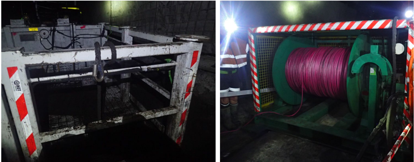
Figure 1 - Rope looped over workbasket handrail (left), and rope spool at conveyor tail (right)
