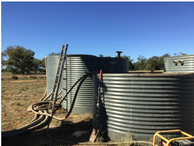
Figure 5 Fluid management system at DCKDH018 using poly tanks to re-circulate drilling fluids
