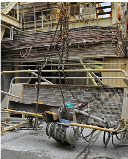
Picture 15. Scene of the incident.
