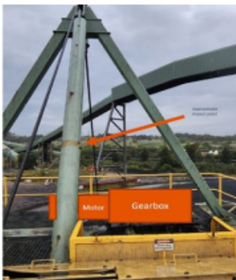
Figure 1: Reclaimer motor and gearbox
