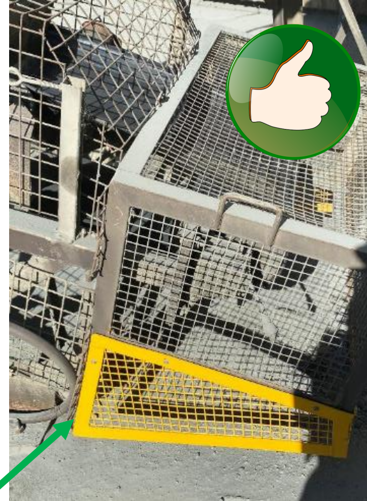
Improved guarding – preventing access to undersides
