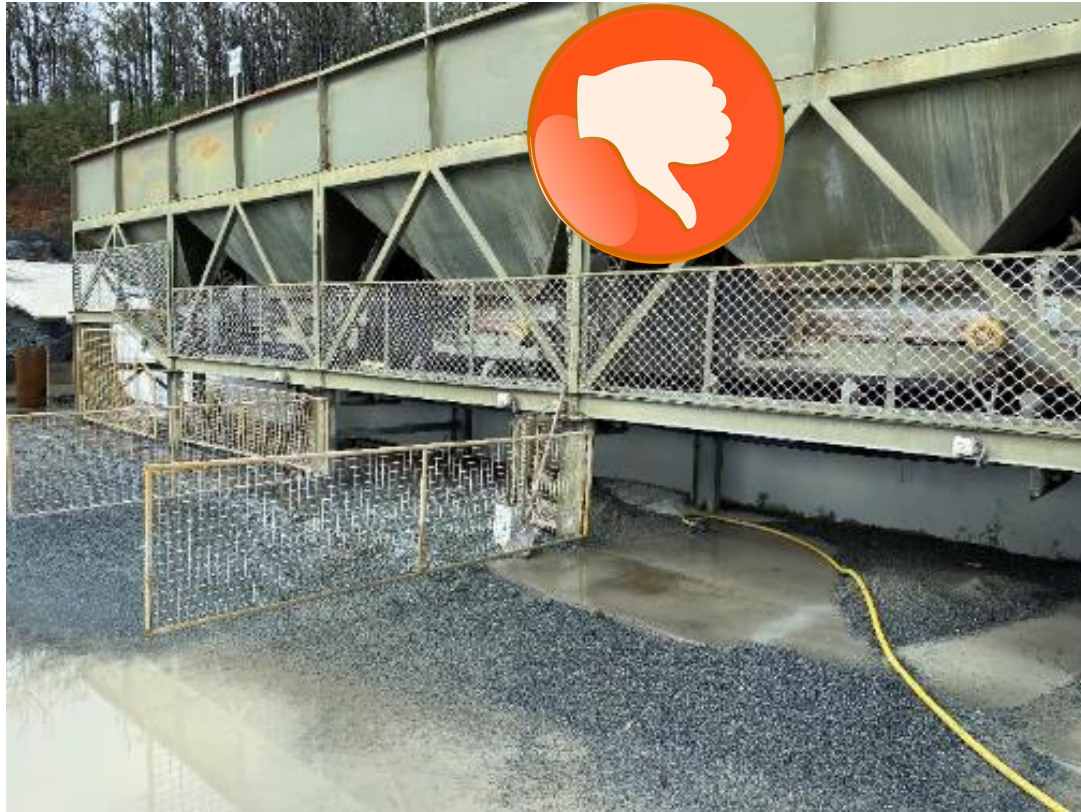
No isolation under conveyor while cleaning
