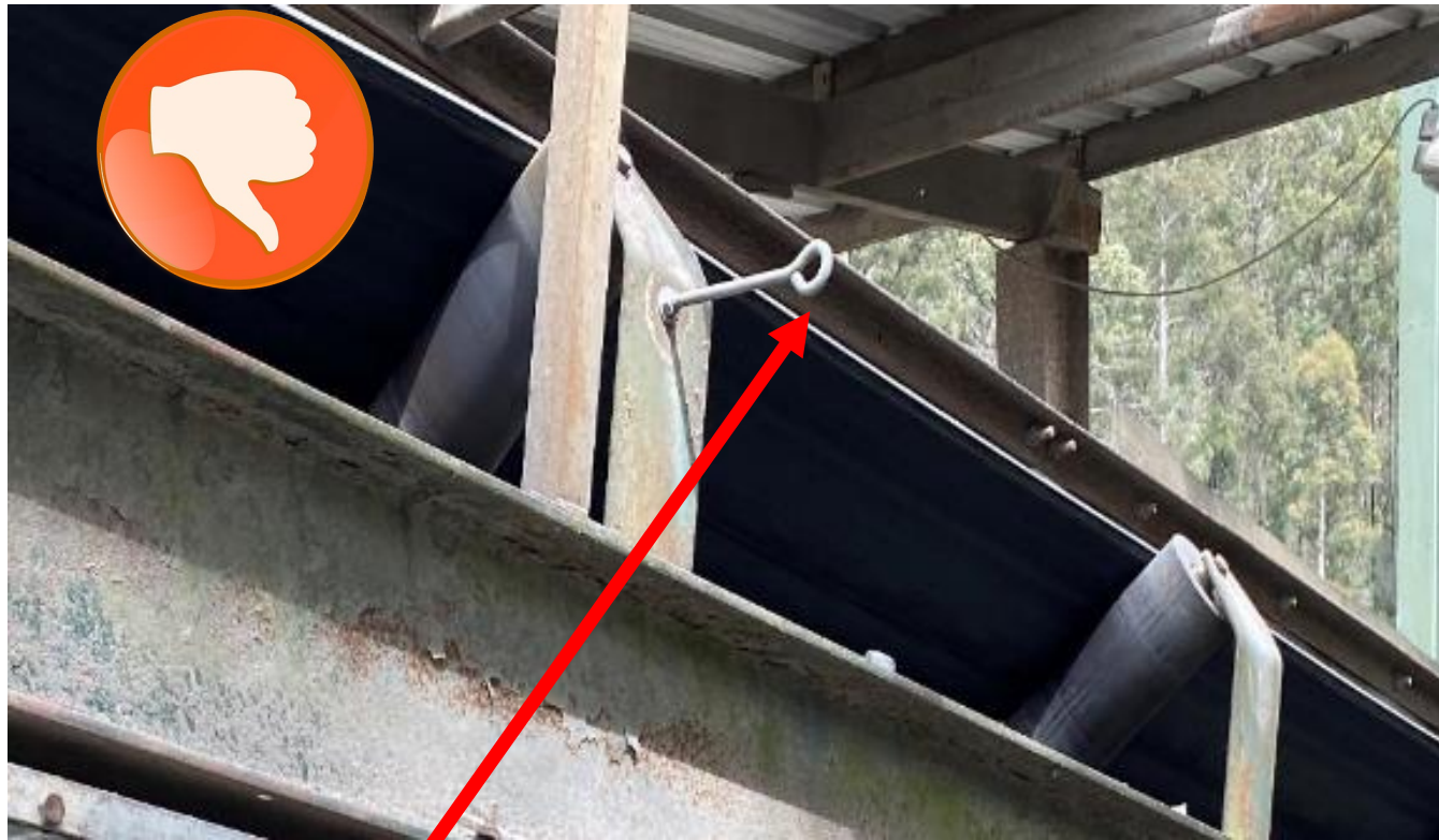
Missing emergency stop lanyard
