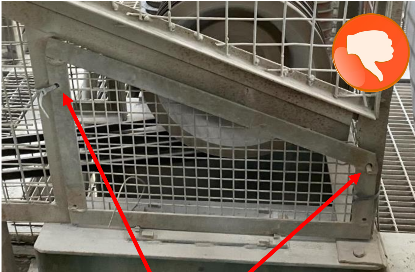
Poor guard security – cable tie and missing nut
