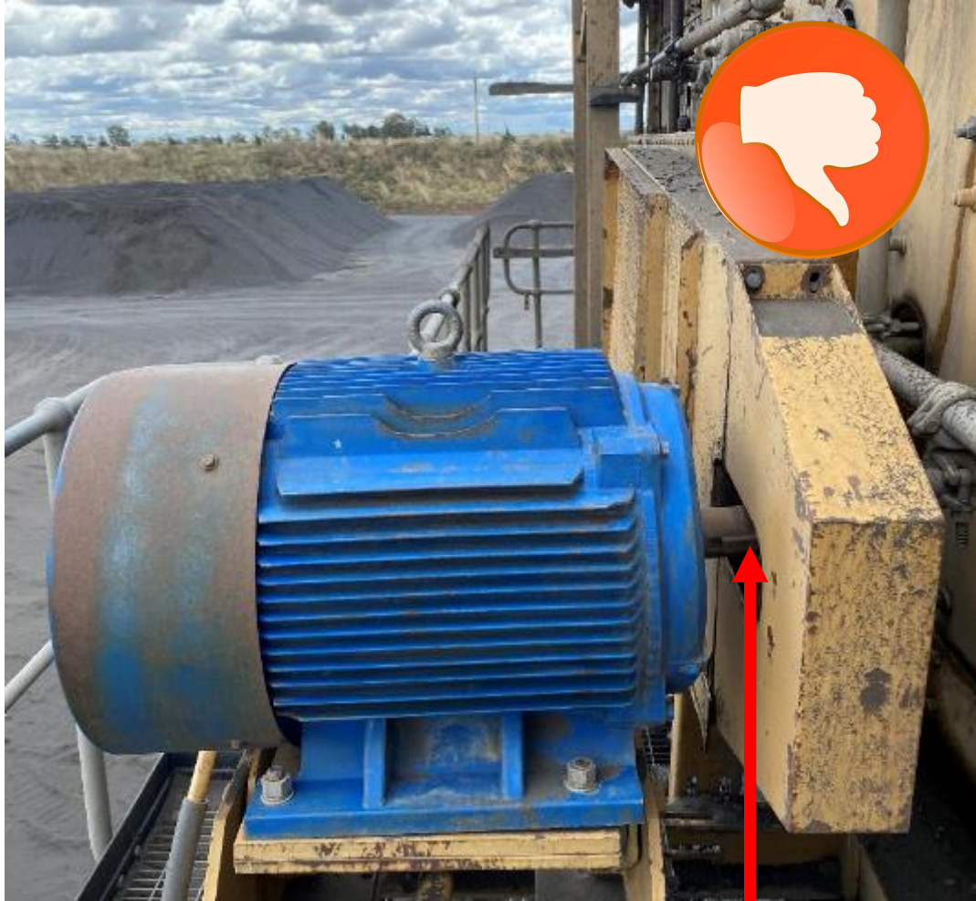
Poor guarding – exposed shaft and keyway
