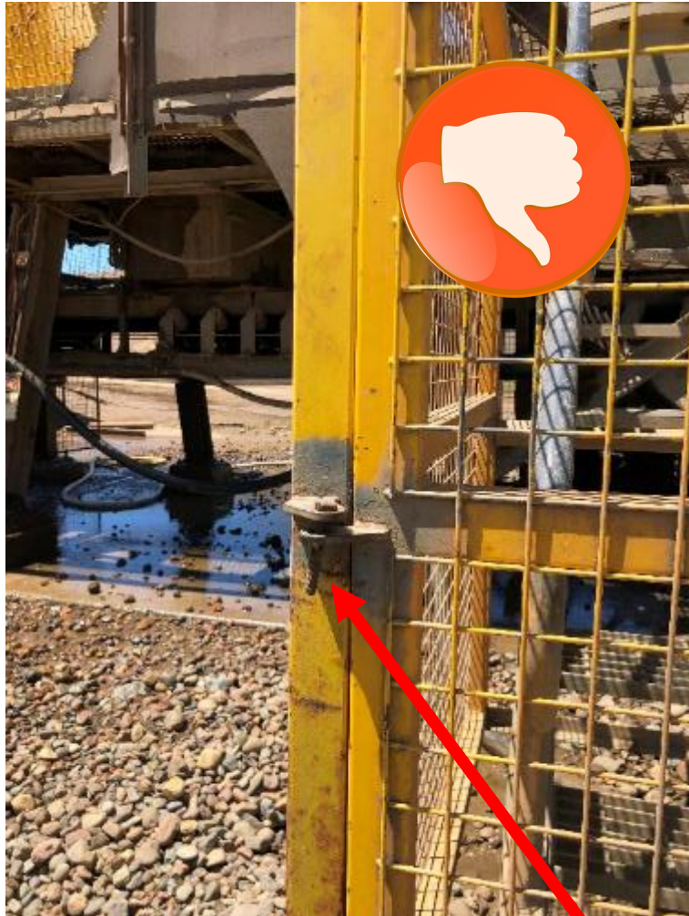
Perimeter fence – not secured (no nut on bolt)
