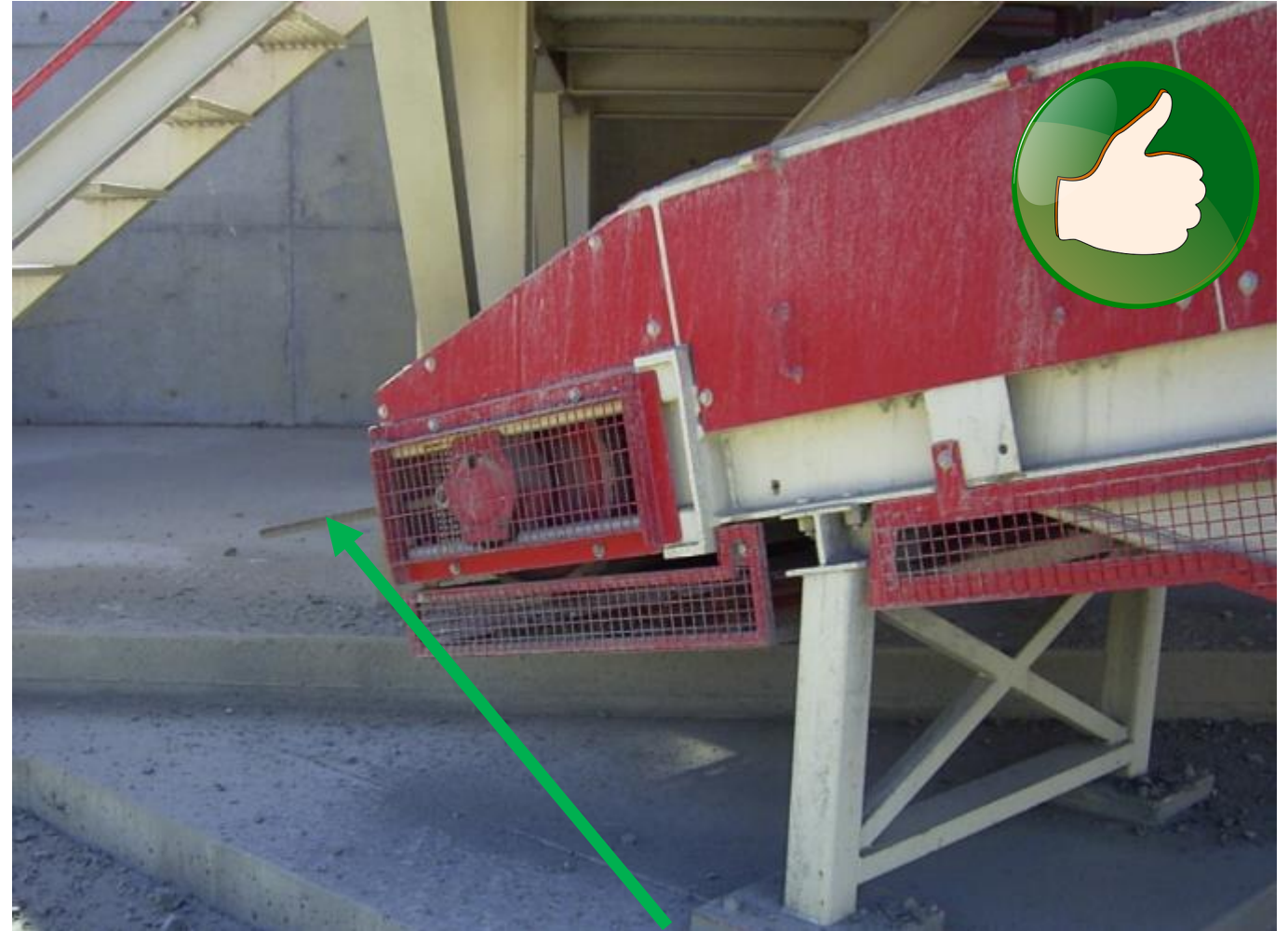
Pulley tensioning external to guard
