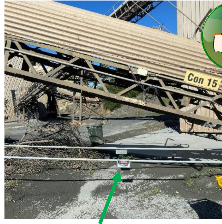
Hard barrier preventing access underneath conveyor with good signposting
