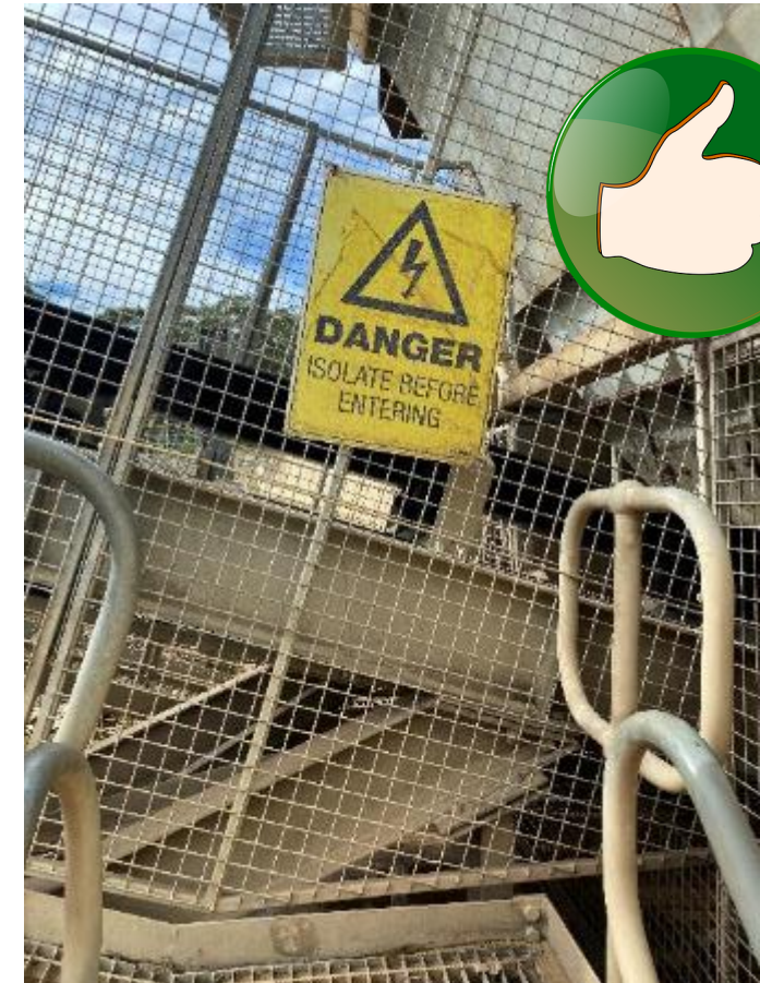
Good signage on guard and full coverage of pinch points
