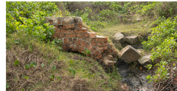
Remains of the old Burwood Colliery railway culvert south of Merewether headland.
