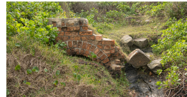
Remains of the old Burwood Colliery railway culvert south of Merewether headland.
