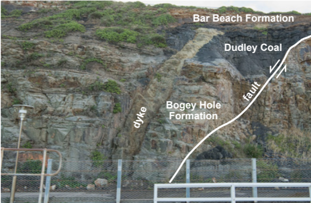
Dyke, fault and joints cross-cutting older sandstone and coal rocks at Newcastle Beach south.
