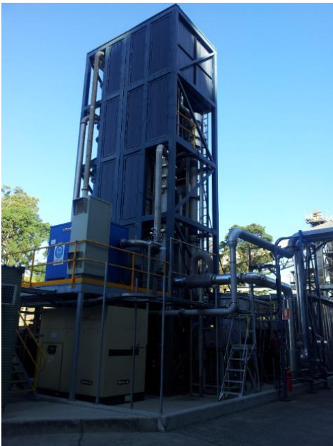
Figure 37 Side view of pilot plant – May 2014
