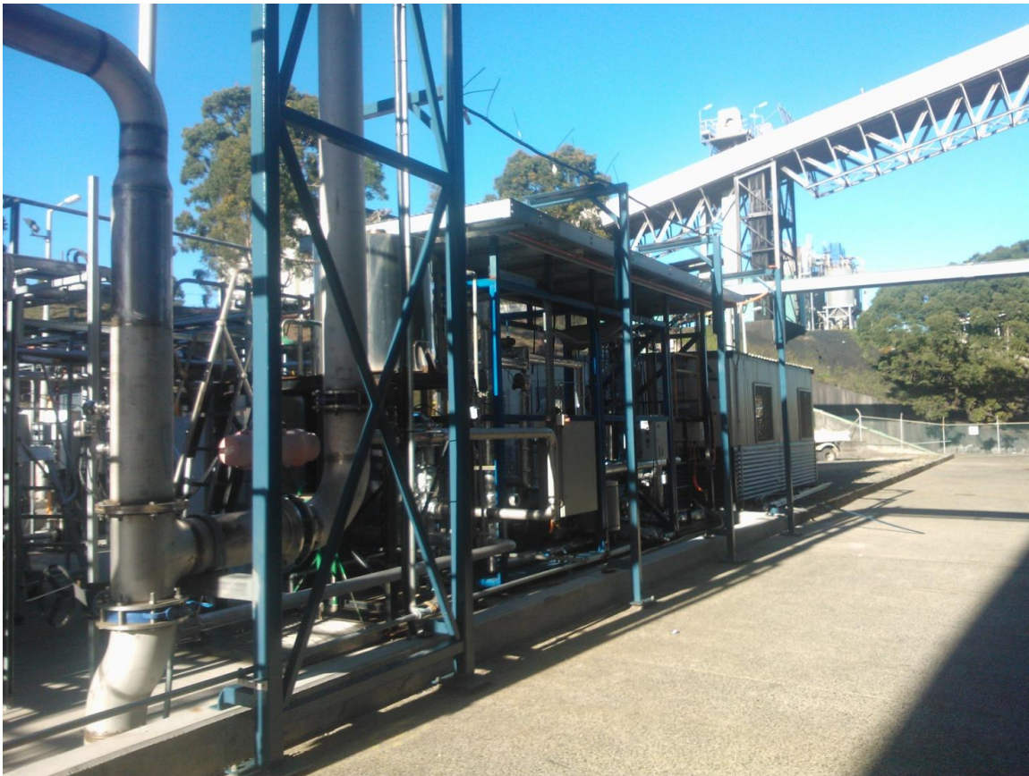
Figure 36 Completed connection to solid sorbent rig and additional electrical and small pipework in the background
