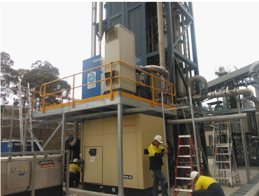
Figure 28 Blower and electrical control cabinet on top of new platform. Compressor below
