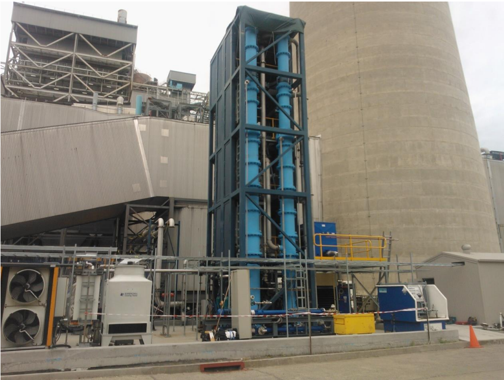
Figure 25 Overall view of plant showing additional pipework, cable trays and high voltage supply shed.
