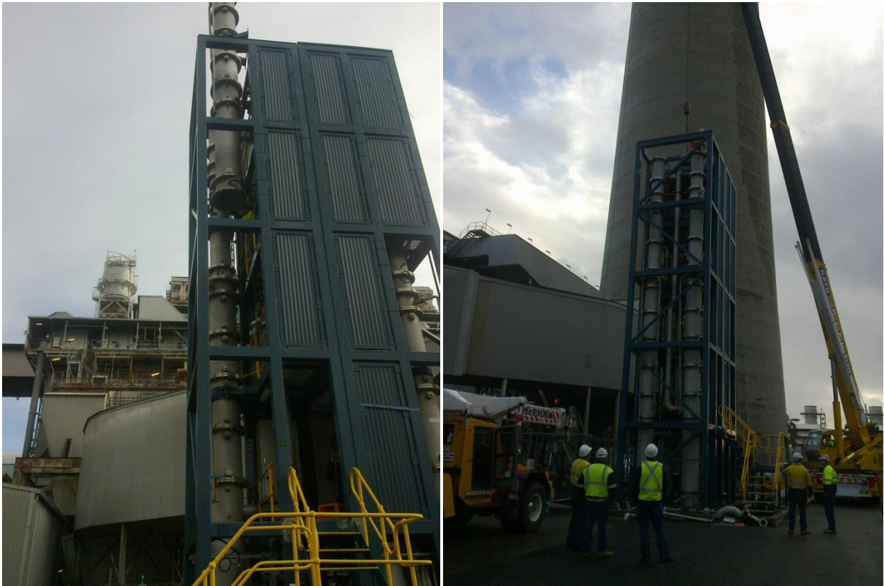
Figure 19 Removal of absorber column for installation of new packing and insulation treatment
