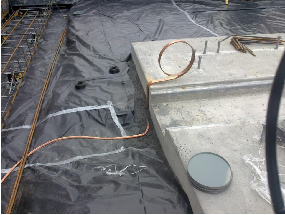
Figure 12 Slab and structure earthing straps
