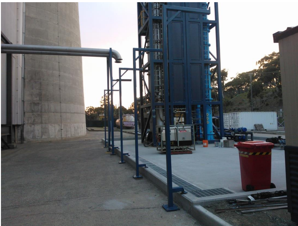
Figure 24 Inlet pipework from the flue gas duct (not connected)
