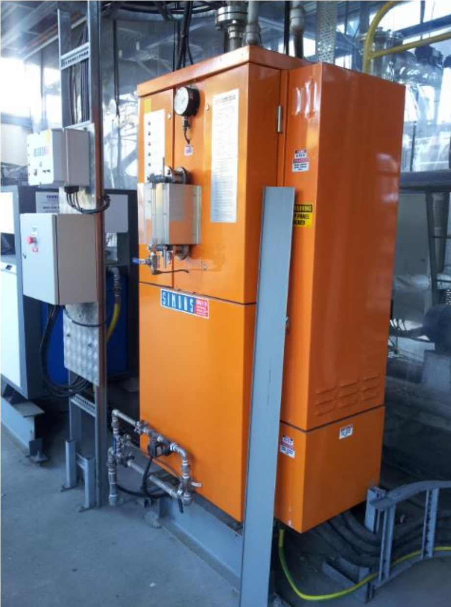
Figure 6 Electric boiler installed
