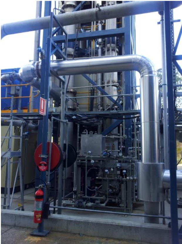
Figure 33 Many runs of hard piping replacing previous flexible hose.
