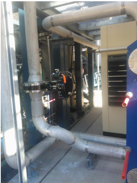
Figure 34 Installation of pipework and new control valve from after cooling heat exchanger
