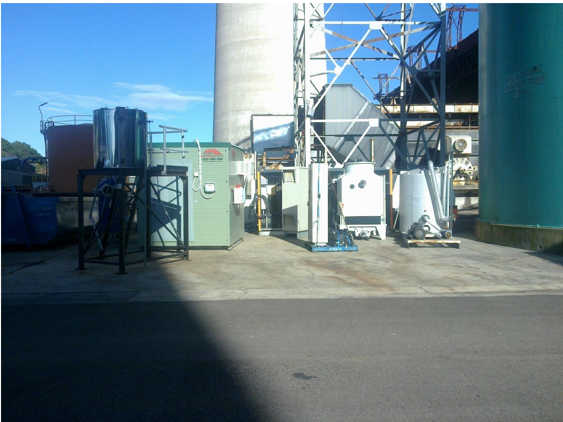
Figure 18 Disconnected ancillary equipment
