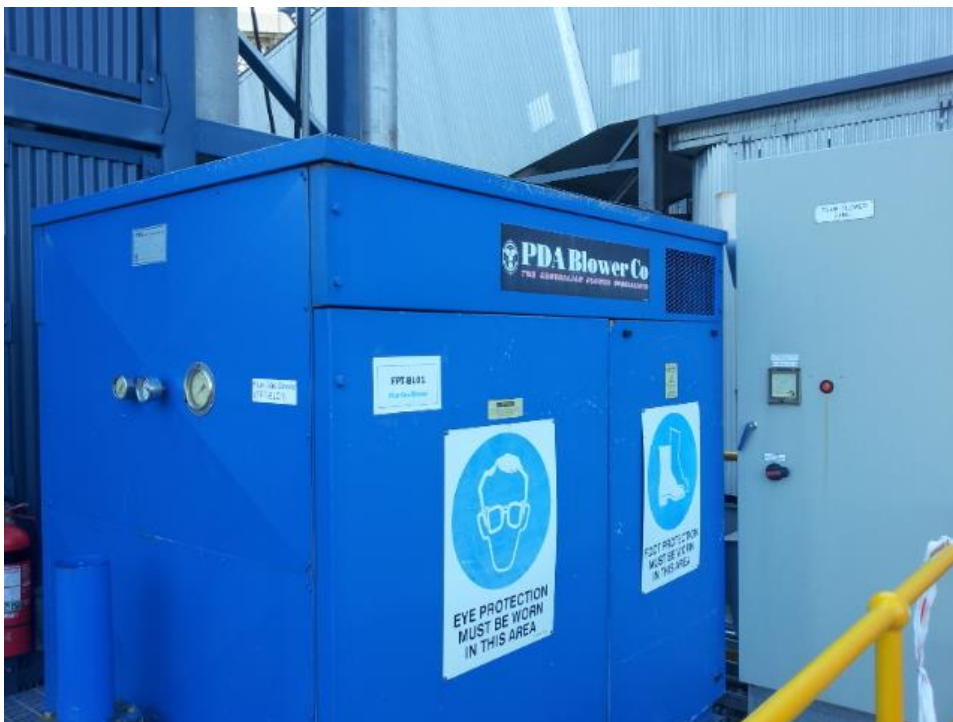
Figure 3 Blower for flue gas
