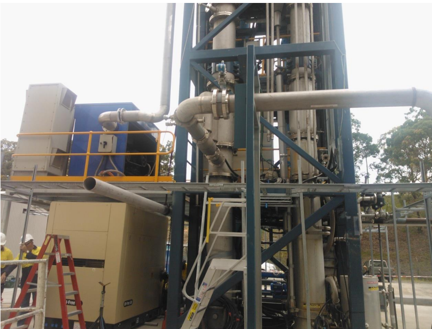
Figure 26 Closer view showing new blower platform, with blower and new compressor in position.
