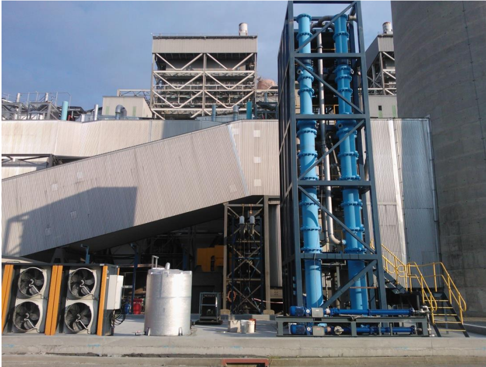
Figure 23 Main pilot plant structure re-assembled with insulated absorber columns in place
