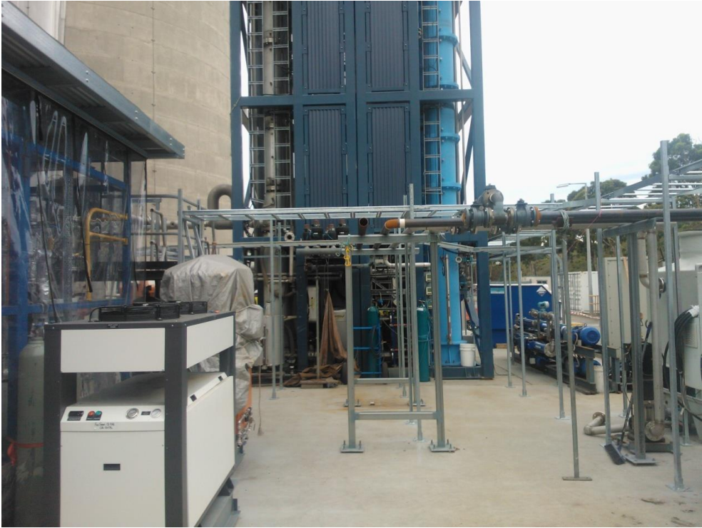
Figure 32 Pipework and cable trays
