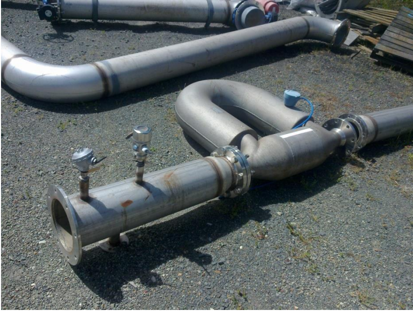
Figure 22 Pipework showing weld corrosion damage
