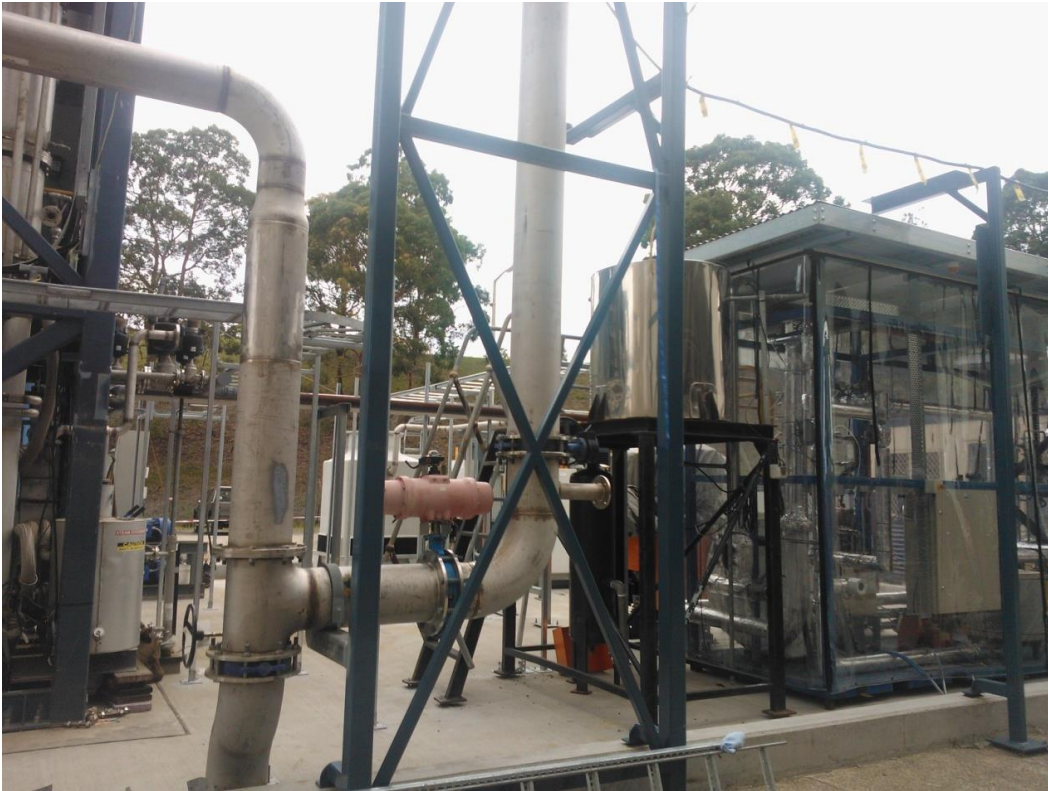
Figure 29 New pipework for blower and flue gas compressor
