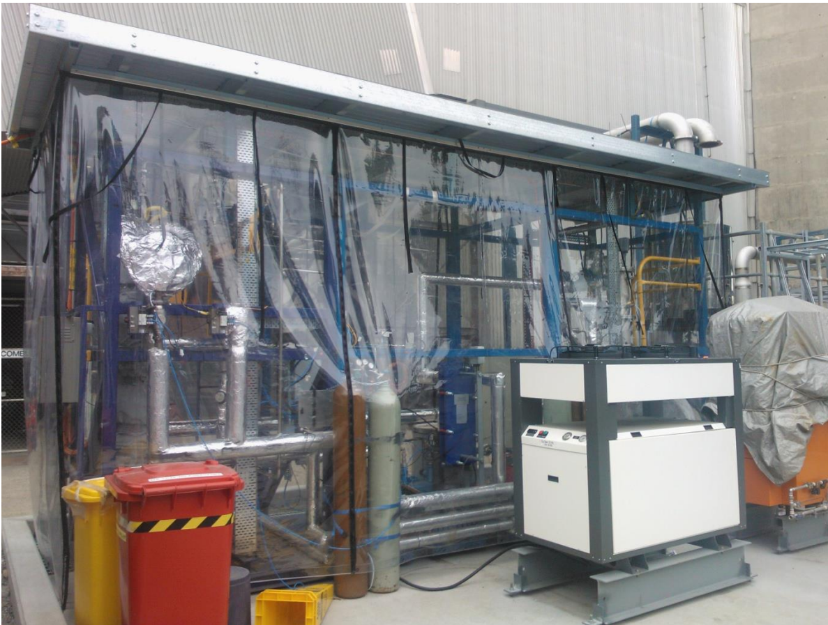
Figure 5 Carbon adsorption plant installed on site
