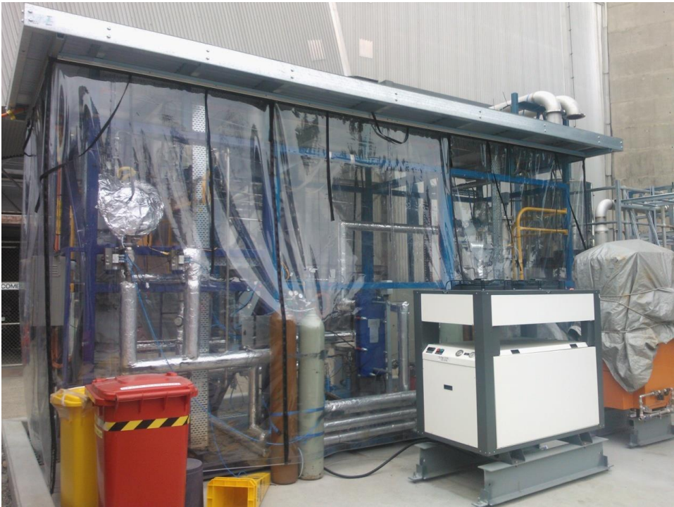
Figure 31 Boiler and chilling unit located in front of solid adsorbent unit
