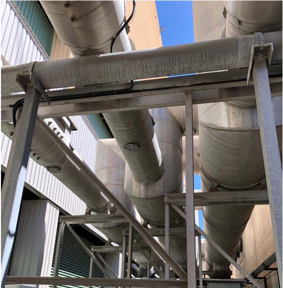
Figure 8.2: Image of Gas-Insulated 23kV feeder lines from the main 23kV bus to auxiliary transformer (smaller gauge gas insulation casing assumed to carry lower-rated 23kV cable).
