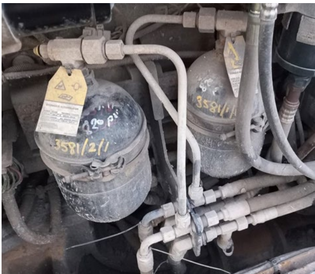
Figure 2 Front and rear brake accumulators
