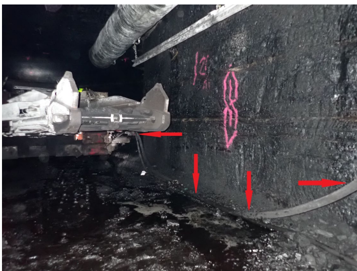
Figure 2 - Trailing electrical cable fixed to miner
