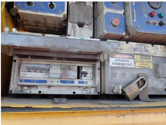
Figure 3– Unsecured LV electrical protection devices – accessible by non-electrical workers
