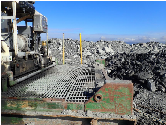
Figure 1– Fall from Heights risk - sled style lighting plant
