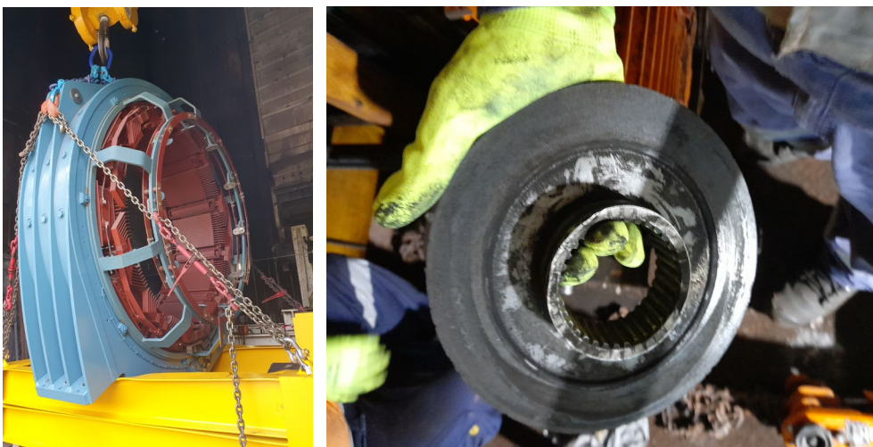
Figure 3 - Motor stator (left) - restrained after fall and brake disc (right)
