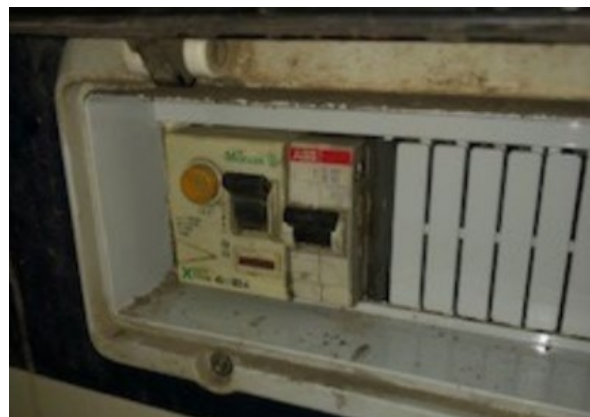
Below: Circuit breaker and control cabinet.
