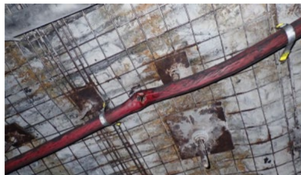
Below: Damaged HV electrical cable hanging from roof of drive.
