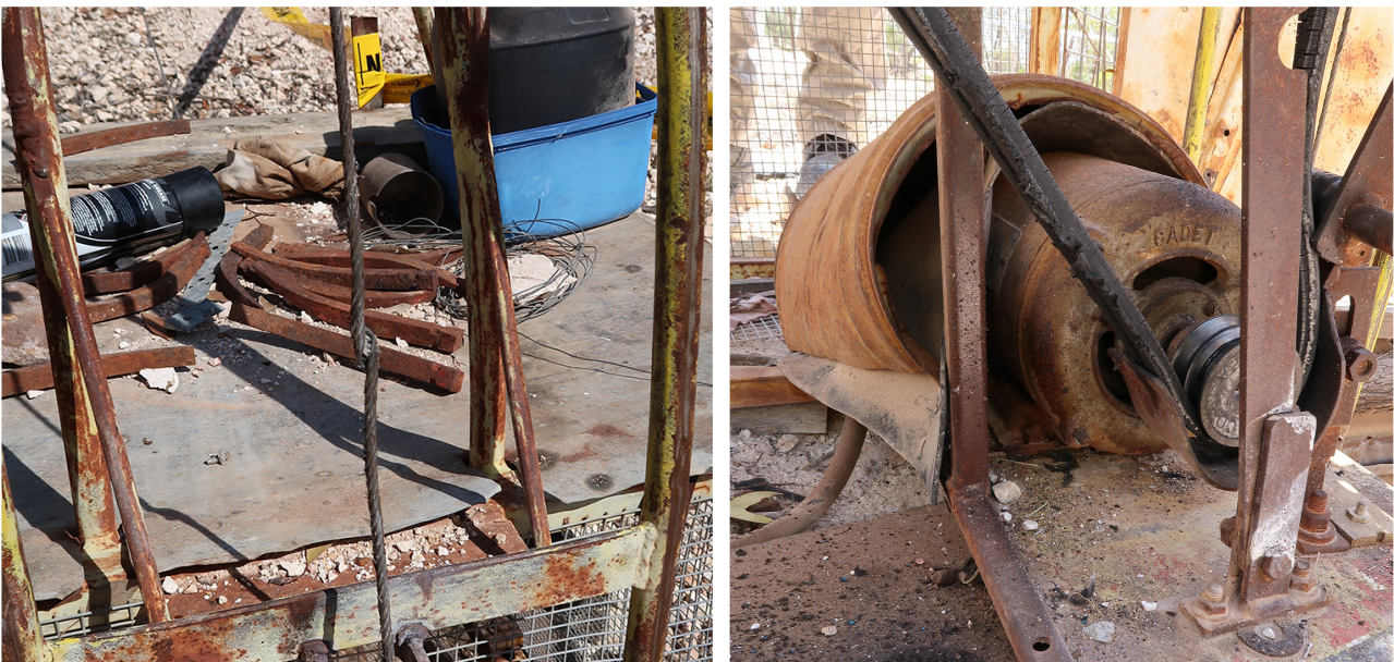
Figure 14: Wear and tear observed on wire cable and vee belt
