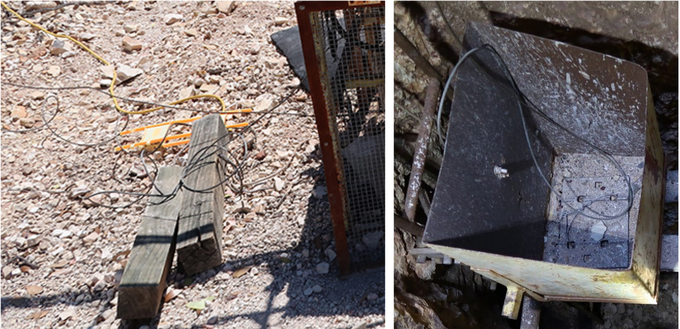
Figure 13: Excess wire spooling at the surface and in the bucket
