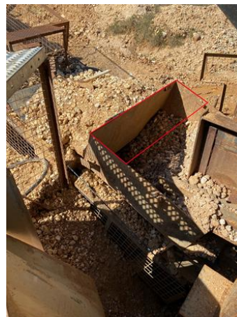
Figure 2: Chute where worker became buried
