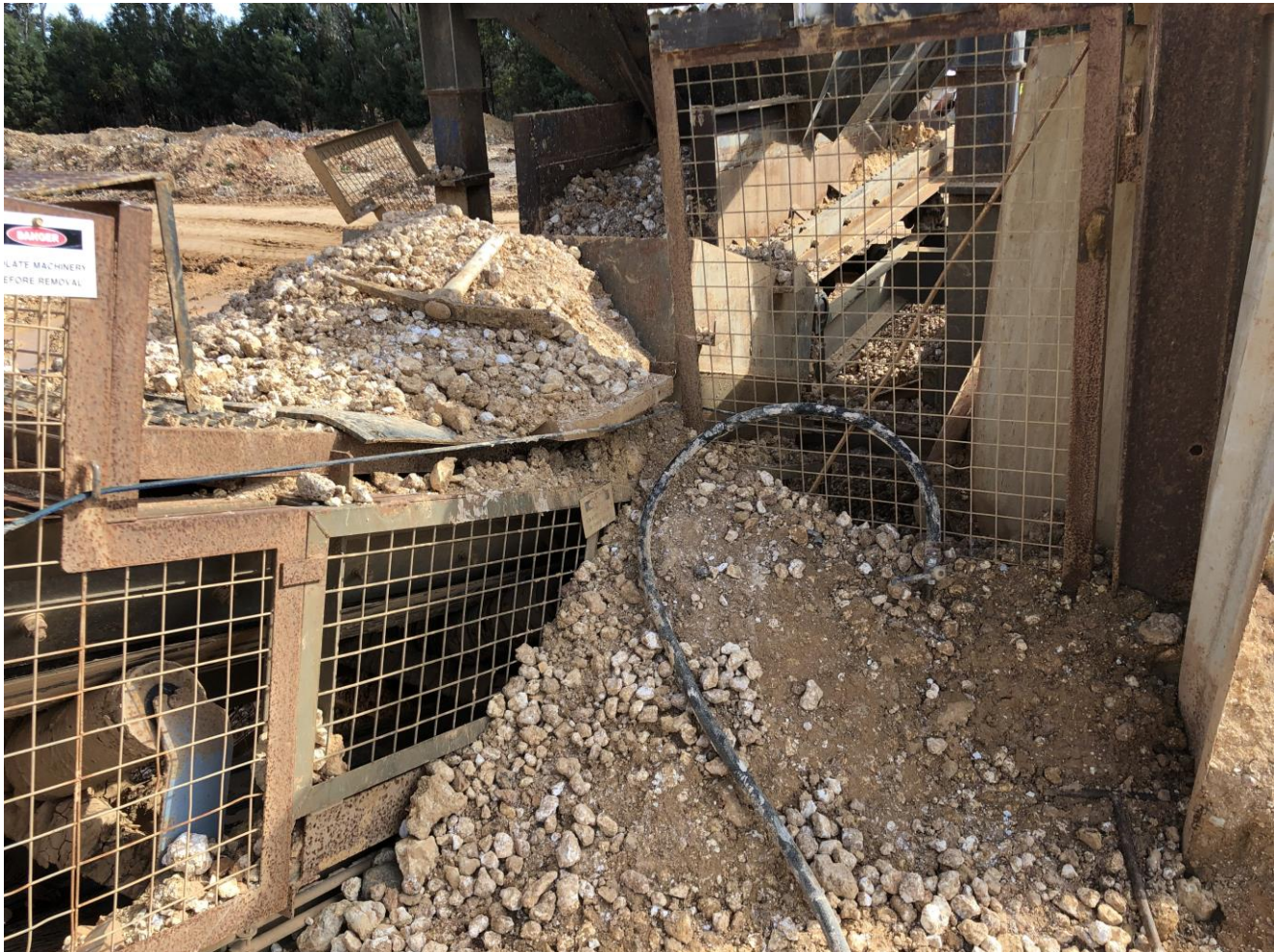
Figure 3: Build-up of material next to the PS25 conveyor which allowed the worker to access the top of the conveyor guard
