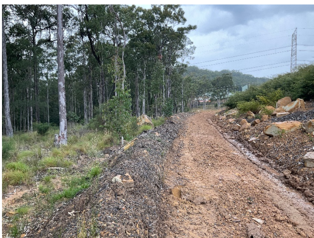
Figure 1. Mulched drainage control bund around stockpile
